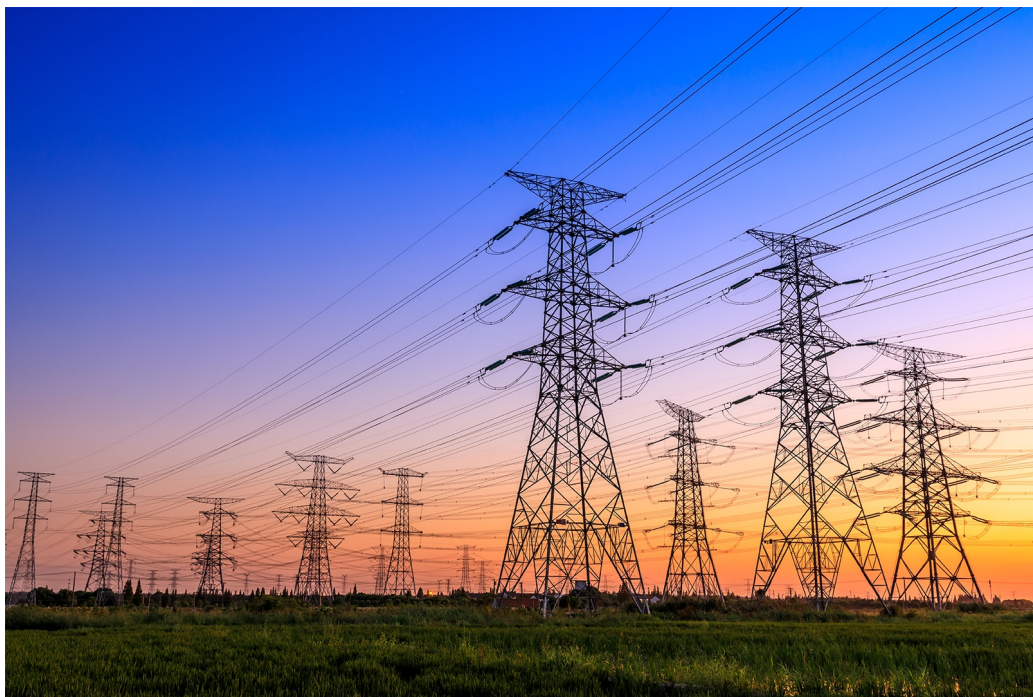
Mynd 1: Háspennulínur Sjá: What is Electricity Price Volatility?
